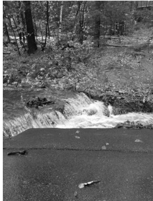
Shoulder damage over a driveway culvert on Watson Pond Road
